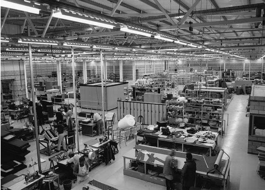
Figure 3.7.1 Factory lighting where fine work is carried out and colour rendering is important, making use of reflector luminaires with tubular fluorescent lamps. (Courtesy Lighting Industry Federation)
