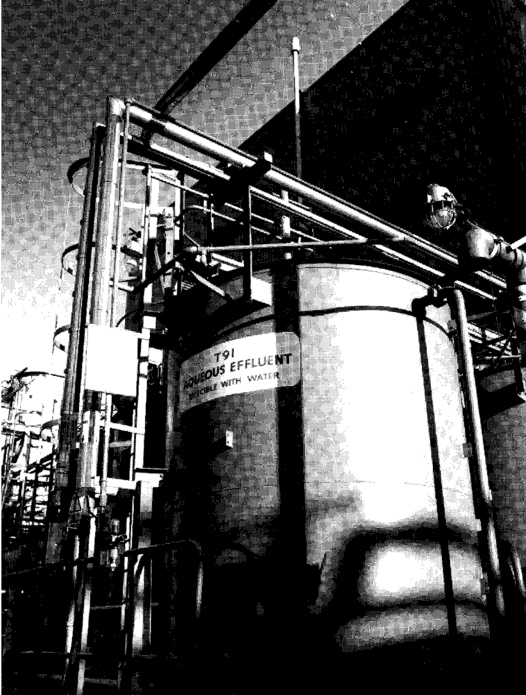
Figure 4.7.4 Storage tank for non-flammable liquids. (Courtesy Rhône-Poulenc-Rorer)
